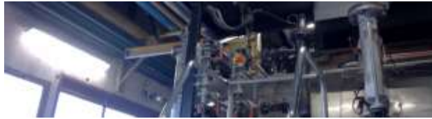
Food & Beverage Process Piping
