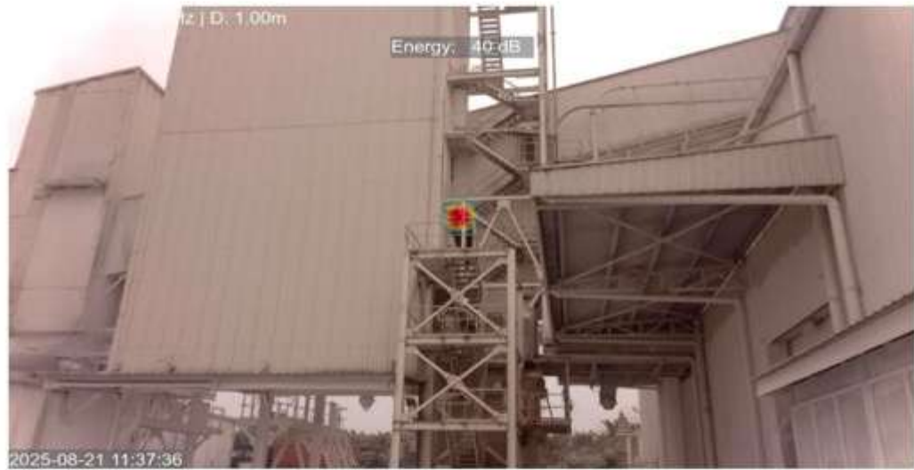
Walk close to the leaks points about 9m close to leak source. Sound energy become higher 40dB
