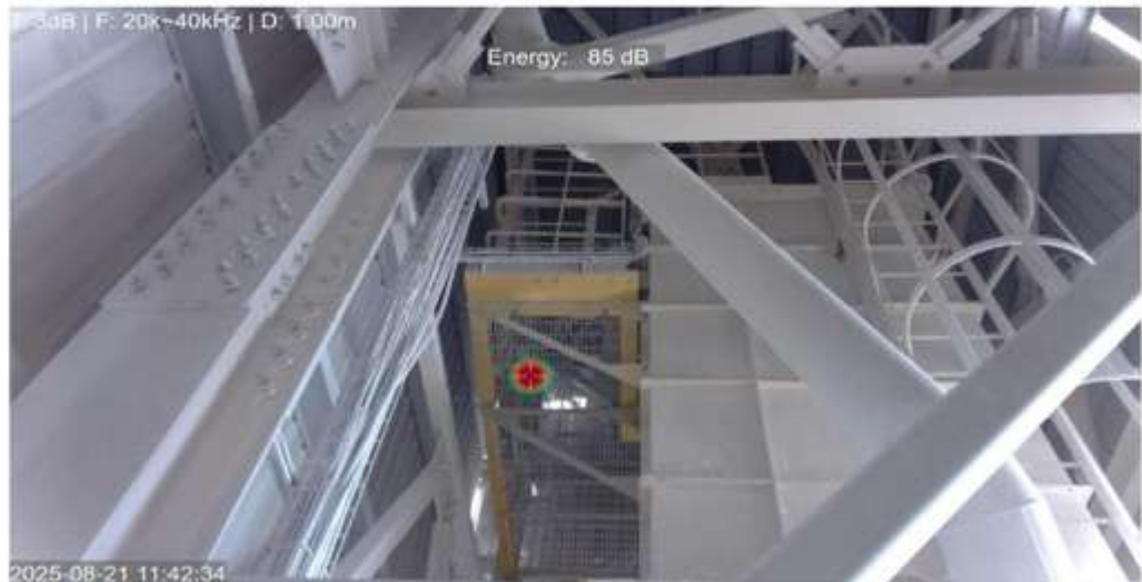
Enter the building and climb up to detects the exact leaks. Sound energy are rated at 85dB
